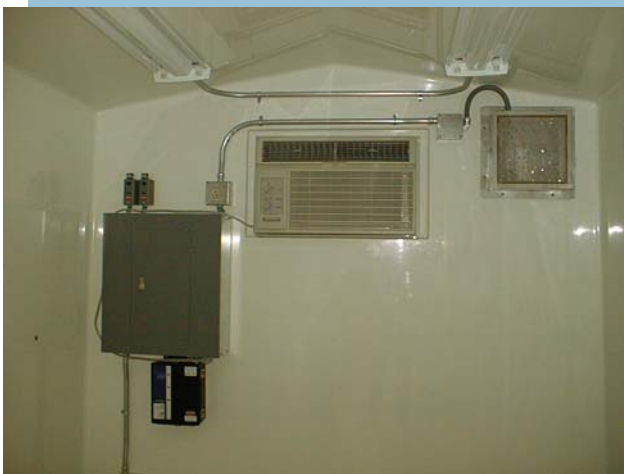
Air Conditioner or Heat Pump
